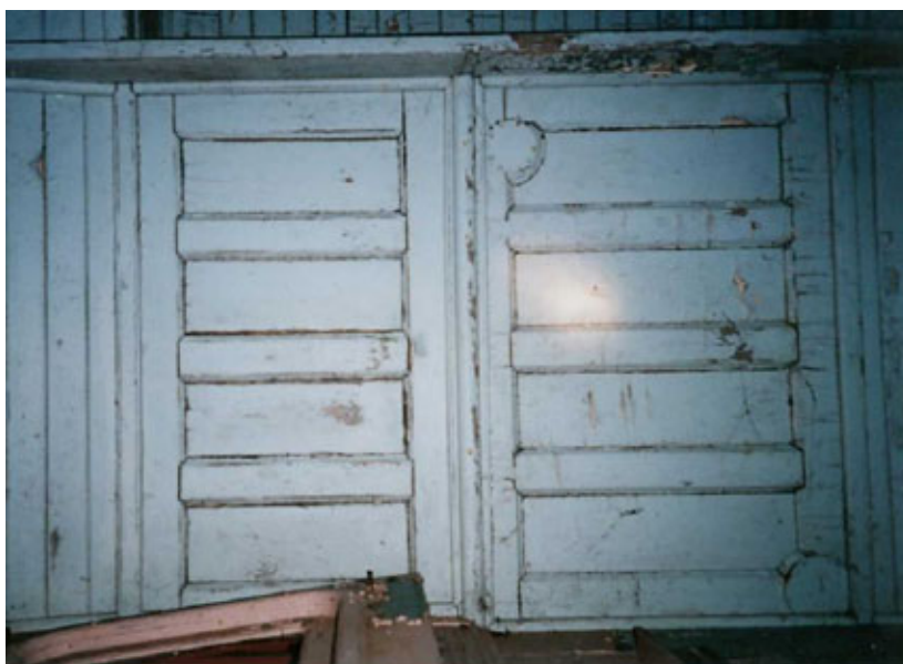
Vestibule ceiling (left), WC ceiling (right) and the end door slightly open at the bottom.
